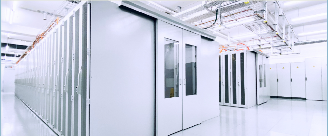
Ventilated customer racks (rear) with separate fiber and copper cable trays above. Central MMR/ODF racks (front).
