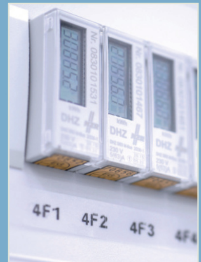
Certified electricity meters per customer and circuit for monitoring and billing purposes.
